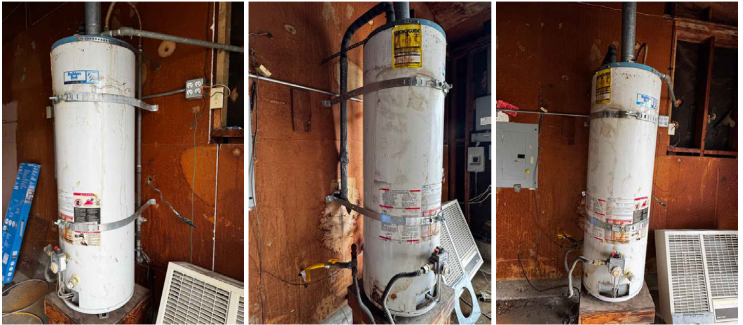
Water heater with seismic straps installed
