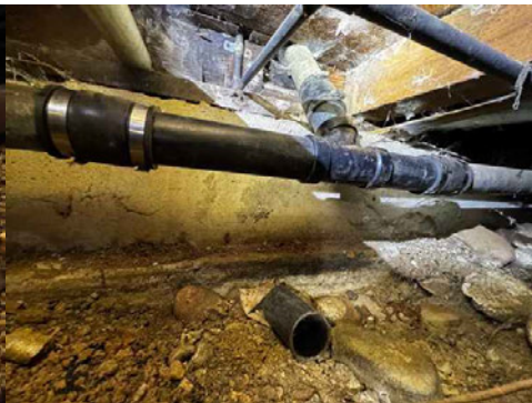
Kitchen drain line repair utilizing unshielded coupling (not consistent with standard above-ground installation practices)
