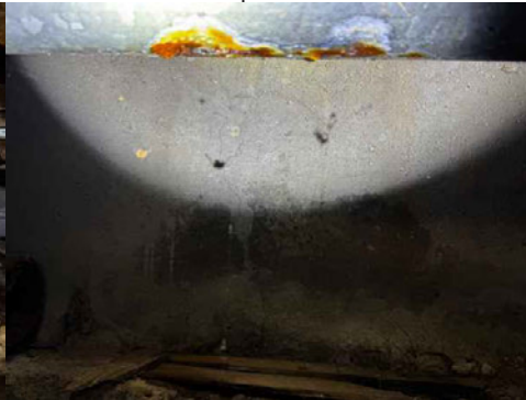
Kitchen drain line: Active leak at electrolysis <12" downstream of repair site
