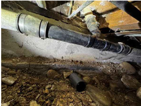
Kitchen drain line repair utilizing unshielded coupling (not consistent with standard above-ground installation practices)
