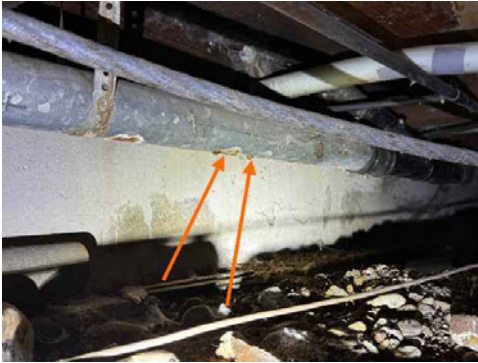
Kitchen sink drain line leaking >12" downstream of repair
