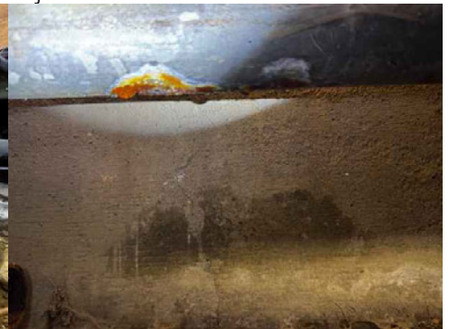
Active leak caused by electrolysis <12" downstream (east) of kitchen drain line repair
