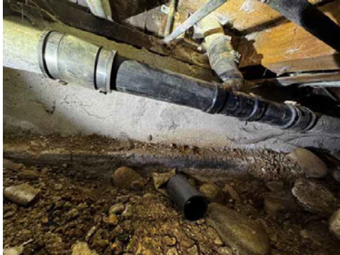
Kitchen drain line repair utilizing unshielded coupling (not consistent with standard above-ground installation practices)
