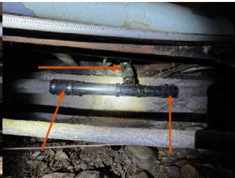
Unshielded couplings used for drain line coupling in crawl space
