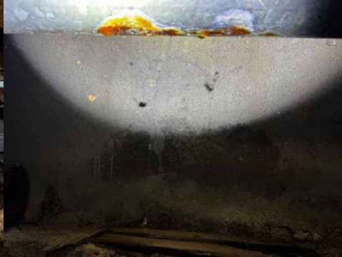
Kitchen drain line: Active leak at electrolysis <12" downstream of repair site
