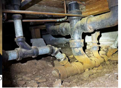
Soil stack with water running: No master tub leaks; no ABS and P-trap replaced as shown on customer invoice
