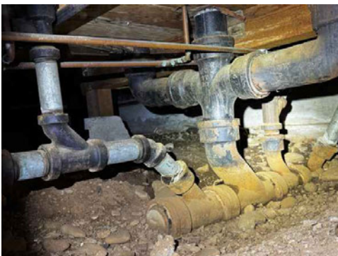
Soil stack with water running: No master tub leaks; no ABS and P-trap replaced as shown on customer invoice
