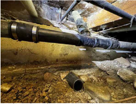
Kitchen drain line repair utilizing unshielded coupling (not consistent with standard above-ground installation practices)
